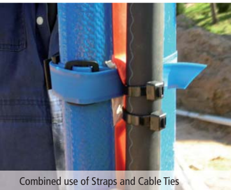
Use of Straps to Fix Cable to Hose
